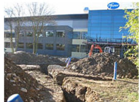
A new energy-efficient geothermal heating and cooling system was installed at the Freiburg, Germany site.
