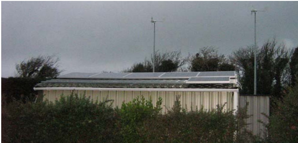
Neil McCarthy's wind turbines and power shed at his home in Ireland
